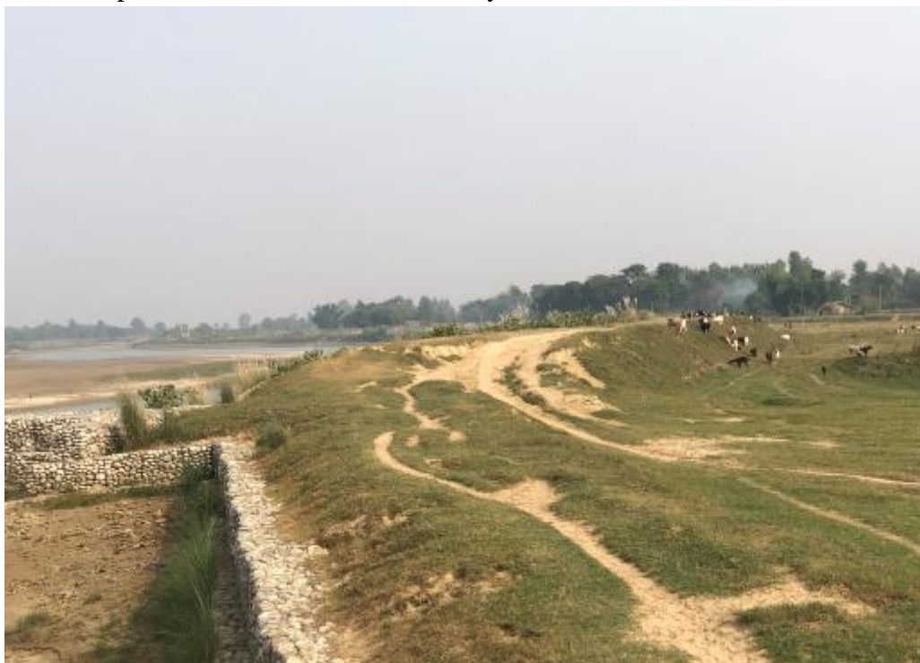
Pic 6: Old eroded embankment at Mohana
